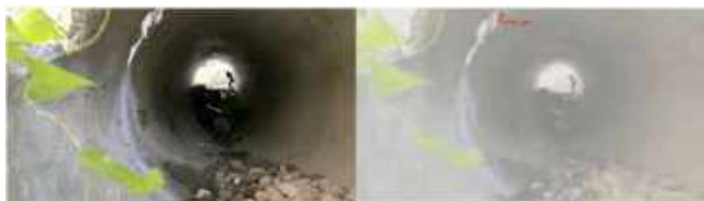
Fig. 6. Input and processed image in daylight is far from damage section
