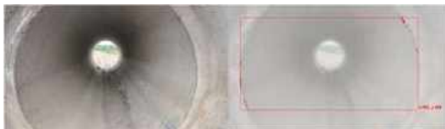
Fig. 8. Input and processed image in daylight with cracks at the junction of pipes.
