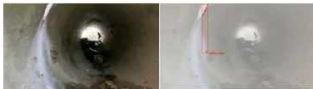
Fig. 7. Input and processed daylight image is closer to the damage section
